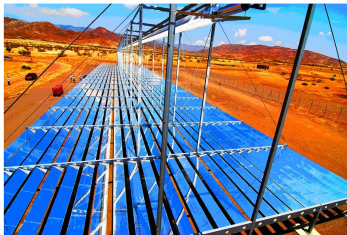
Figure 1-4 Linear Fresnel mirrors at the Plataforma Solar de Almería, Spain [7]
